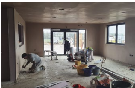
Work is progressing on the interior and exterior areas of Easton's new community centre.
